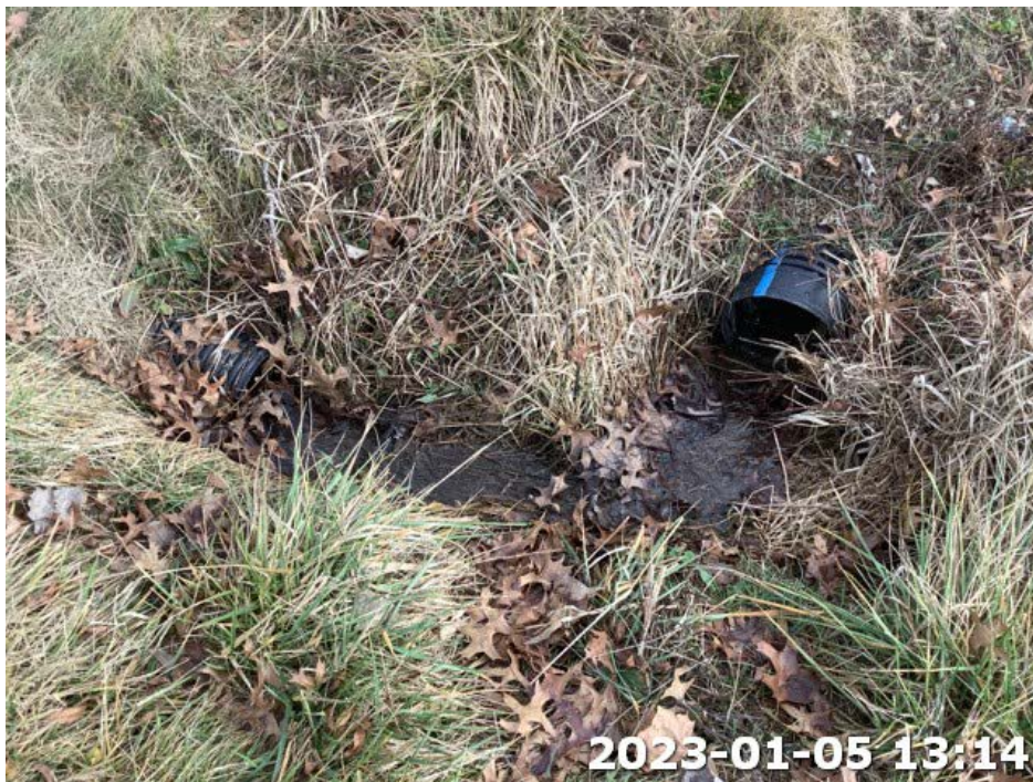
Photograph Location 5. Representative view of existing culvert within the Project area. Photograph taken facing east.
