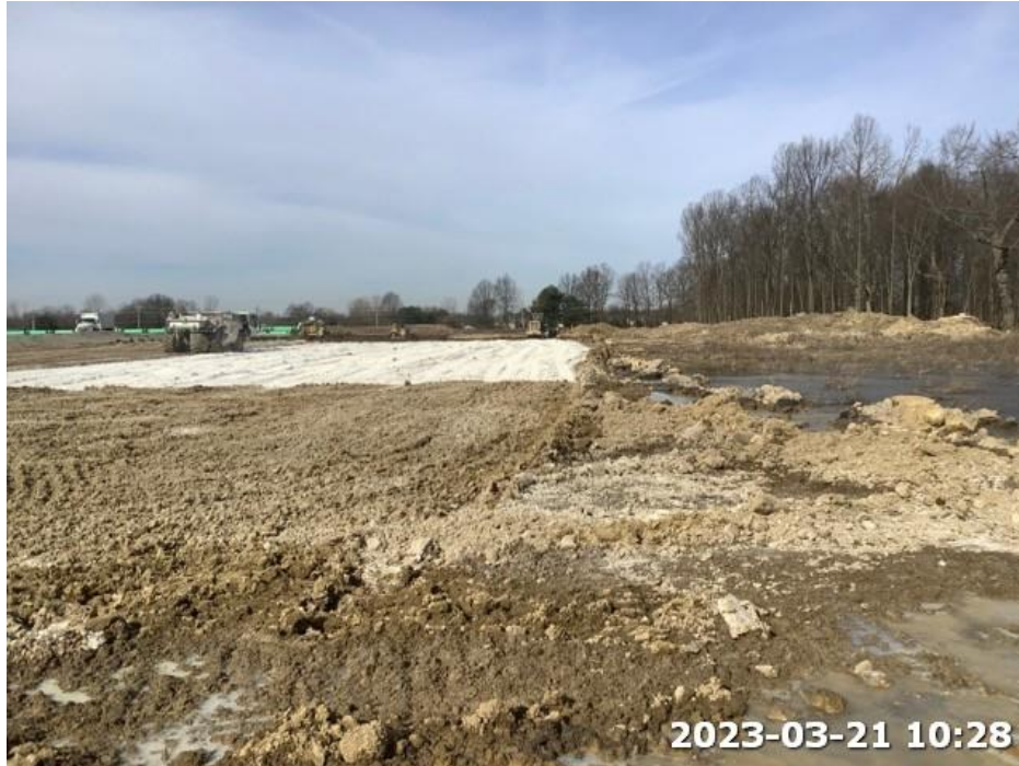
Photo 3. View of grading activities in northeast corner of the Project area. Photograph taken facing west.
