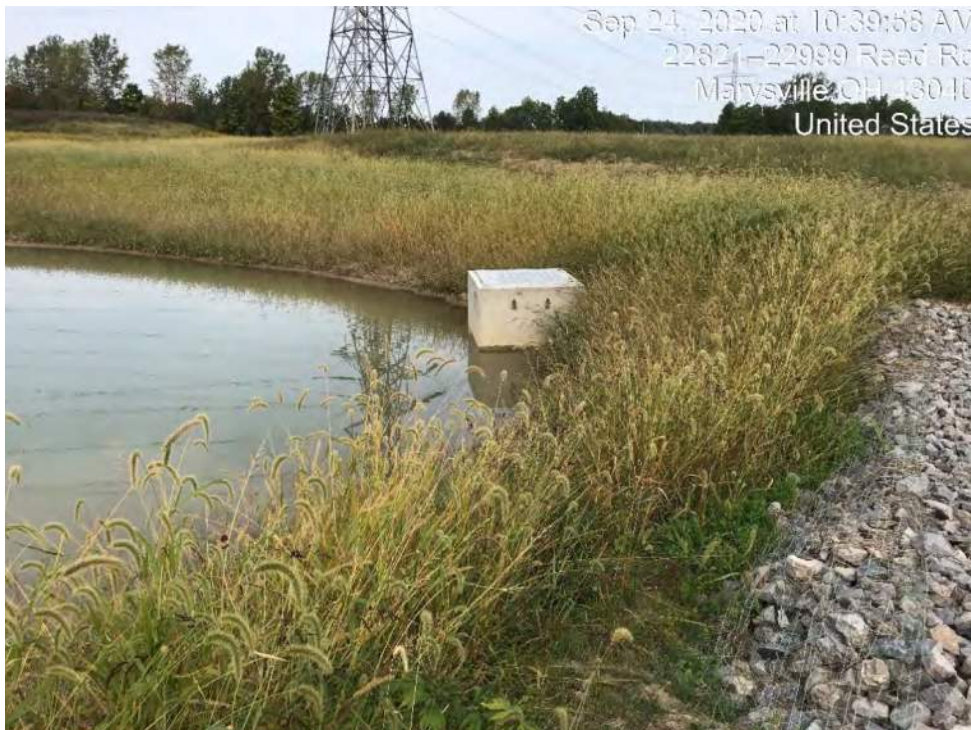
Photo Location 12. View of concrete outfall within the recently constructed stormwater detention basin. Photograph taken facing north.
