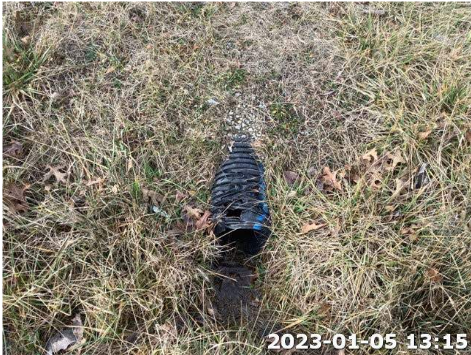
Photograph Location 5. Representative view of existing culvert within the Project area. Photograph taken facing west.
