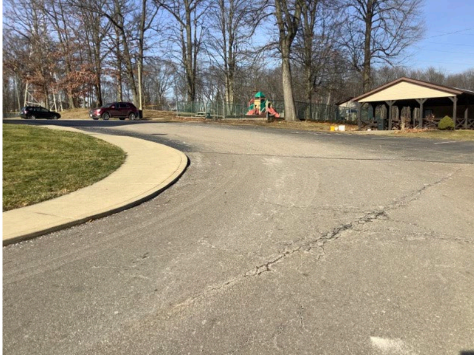
Photograph Location 9. Representative view existing paved road within the Project area. Photograph taken facing north.
