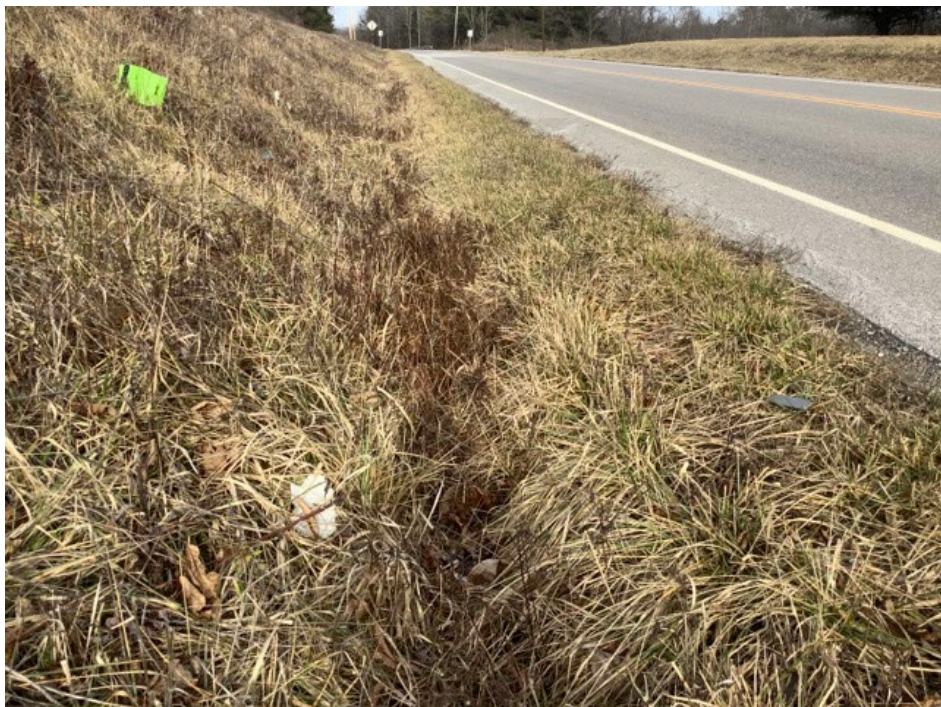
Photograph Location 3. Representative view of an upland drainage feature within the Project area. Photograph taken facing south.
