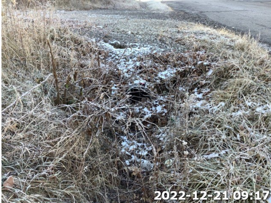
Photograph Location 1. Representative view of an upland drainage feature and existing culvert within the Project area. Photograph taken facing north.
